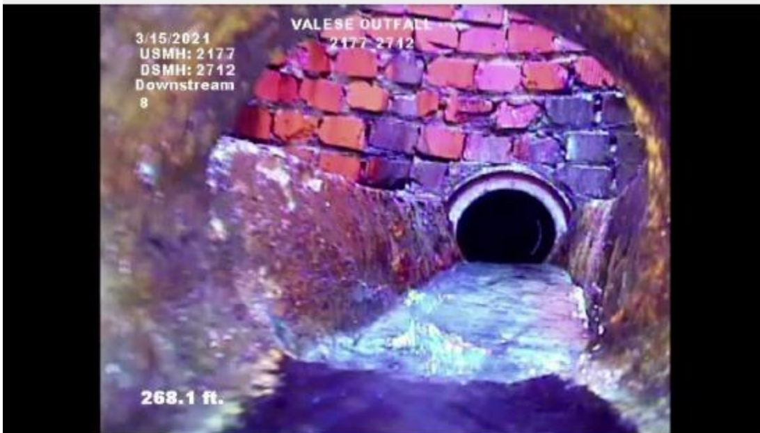
MH 2712 WITH SEVERE LEAK
